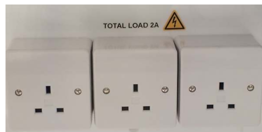
Figure 16: UK Internal Power Sockets
