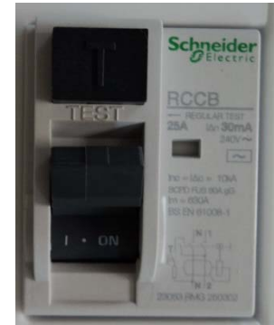
Figure 9: RCCB for the workstation
